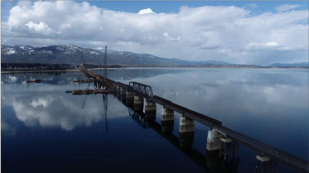
Photograph 1: Drone photograph depicting Project area and start of construction of new bridge crossing looking north.
